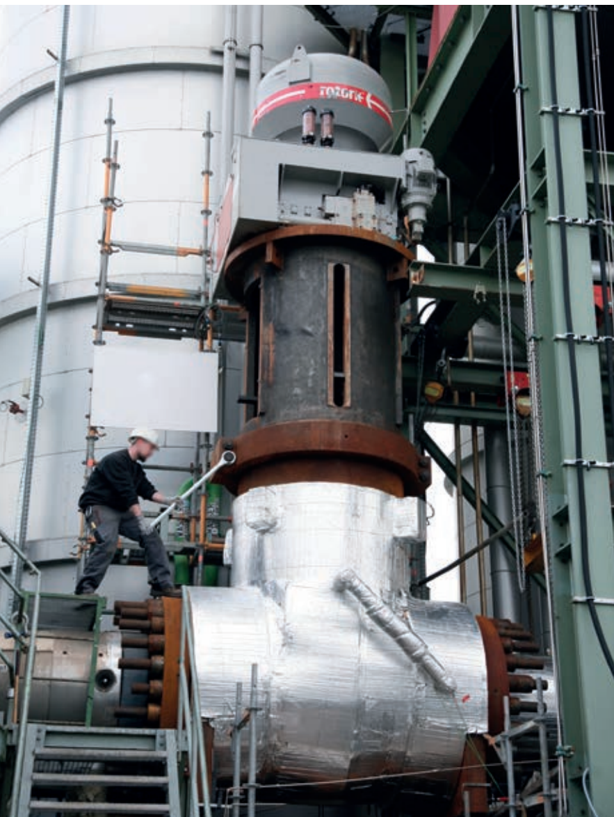
Fig. 10 Large valve in test setup in GAP.
